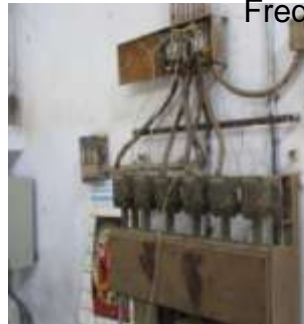
Unsafe Electrical Facilities
