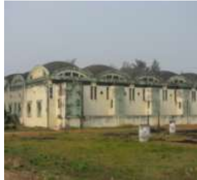
No Prev maintenance of Civil Structures
