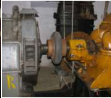
Unsafe Pump couplings
