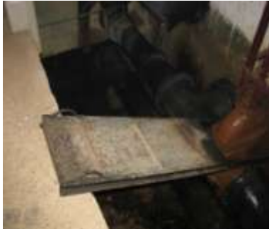
Unsafe working Platforms
