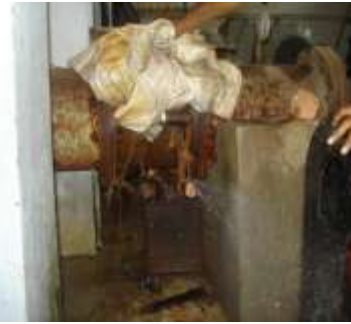
Frequent leaks and poor management of leaks
