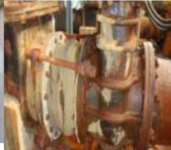
Badly corroded equipments
