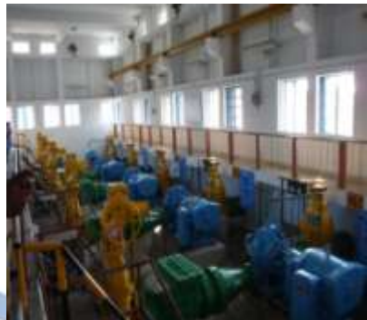
Basudevpur pump house
