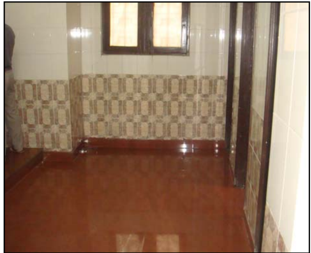
Gent's toilet has adequate space for accessible toilet cubicle by combining existing cubicle and open space
