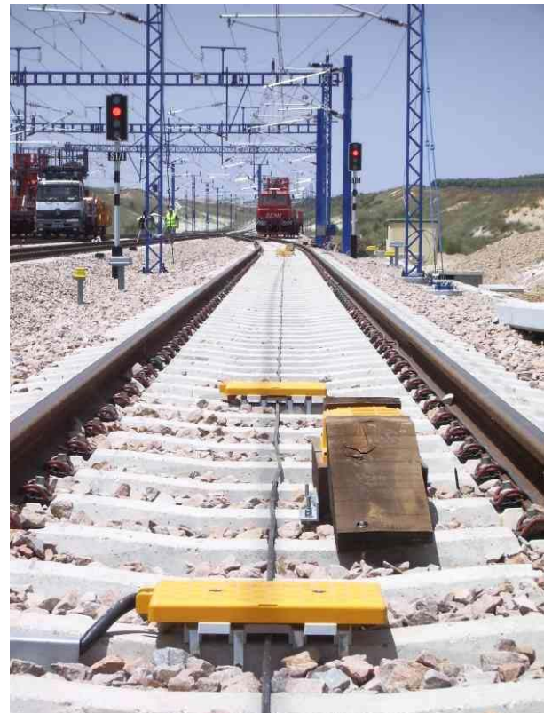
Figure 22 Eurobalise installed in Spain alongside LTB loop and ASFA transponder
