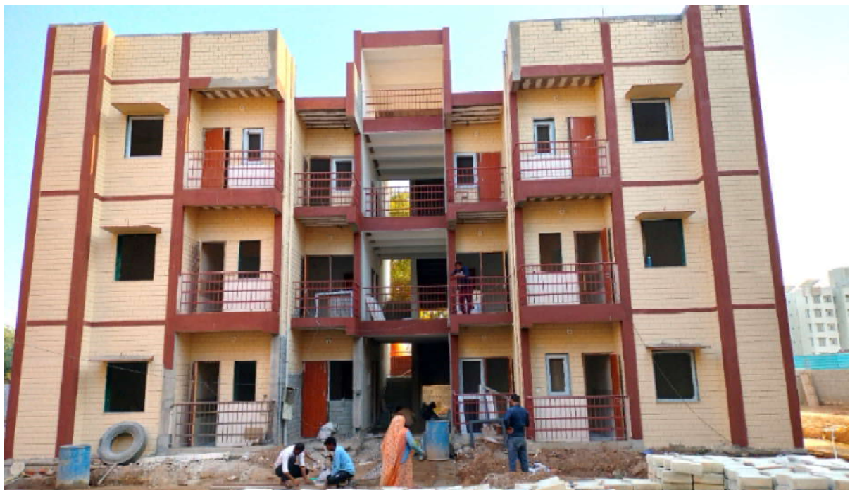
Demonstration Housing Project (PMAY Beneficiaries) under PMAY(U) being constructed by BMTPC using Precast Concrete Construction System - Integrated Hybrid Solution-One at Ahmedabad, Gujarat
