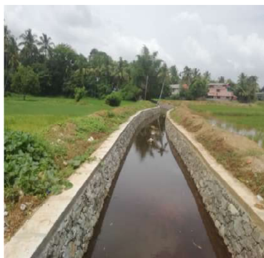
Storm Water Drainage, Thrissur, Kerala
