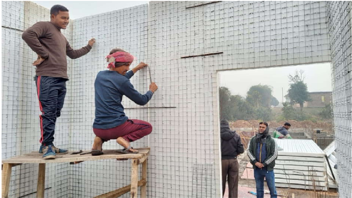
Demonstration Housing Project (for contractual safai karamcharis of GMC and Community Centre) under PMAY(U) being constructed by BMTPC using Light Gauge Steel Structural System - LGSF with V-infill wall at Guwahati, Assam
