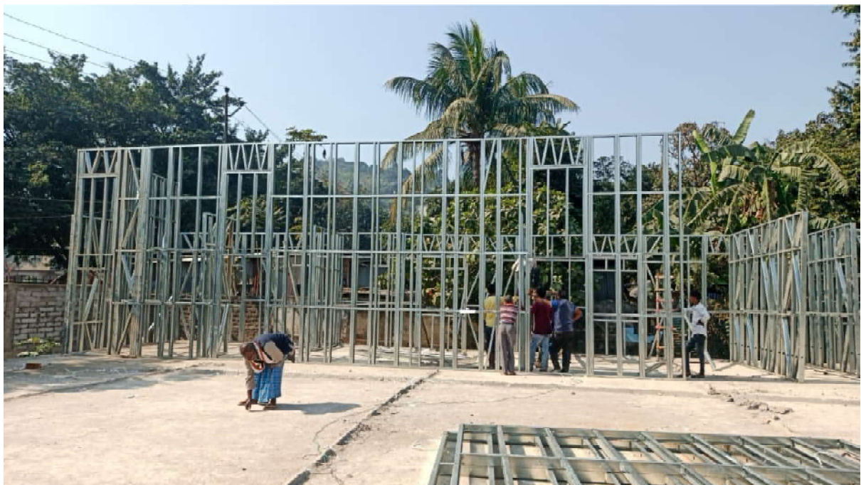
Demonstration Housing Project (Sports Hostel) under PMAY(U) being constructed by BMTPC using Prefabricated Sandwich Panel System - Quik Build 3D Panels at Bhalwal, Jammu, J&K
