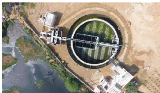
STP at Churu, Rajasthan
