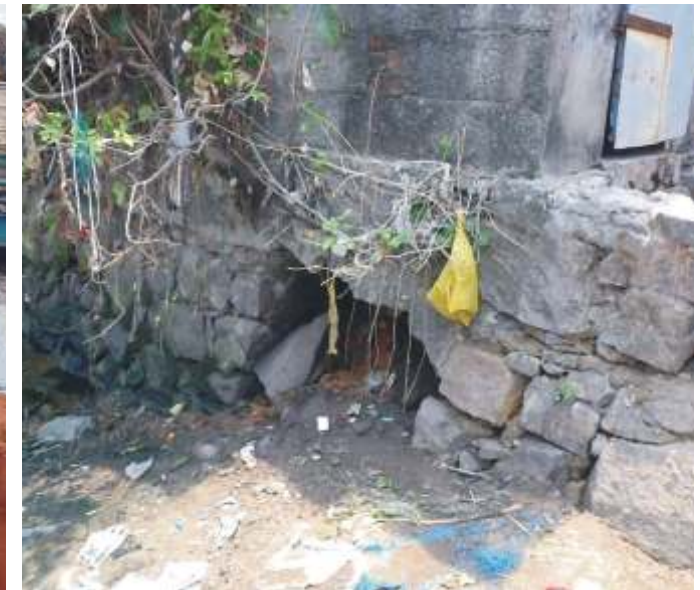
Figure 9: Inadequate septage management
