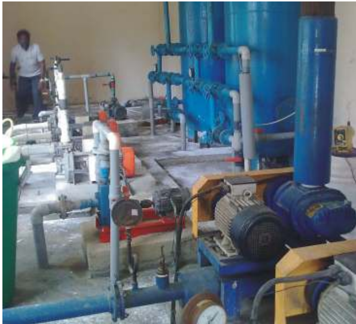
Figure 32: Hi-rise buildings-Inhouse Sewage Treatment facility
