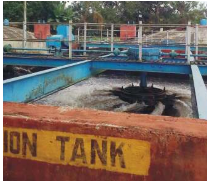
Figure 8: GCDA's sewage treatment plant at Marine Drive
