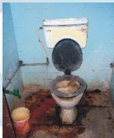
Figure 11(b): Poor condition of CTC
