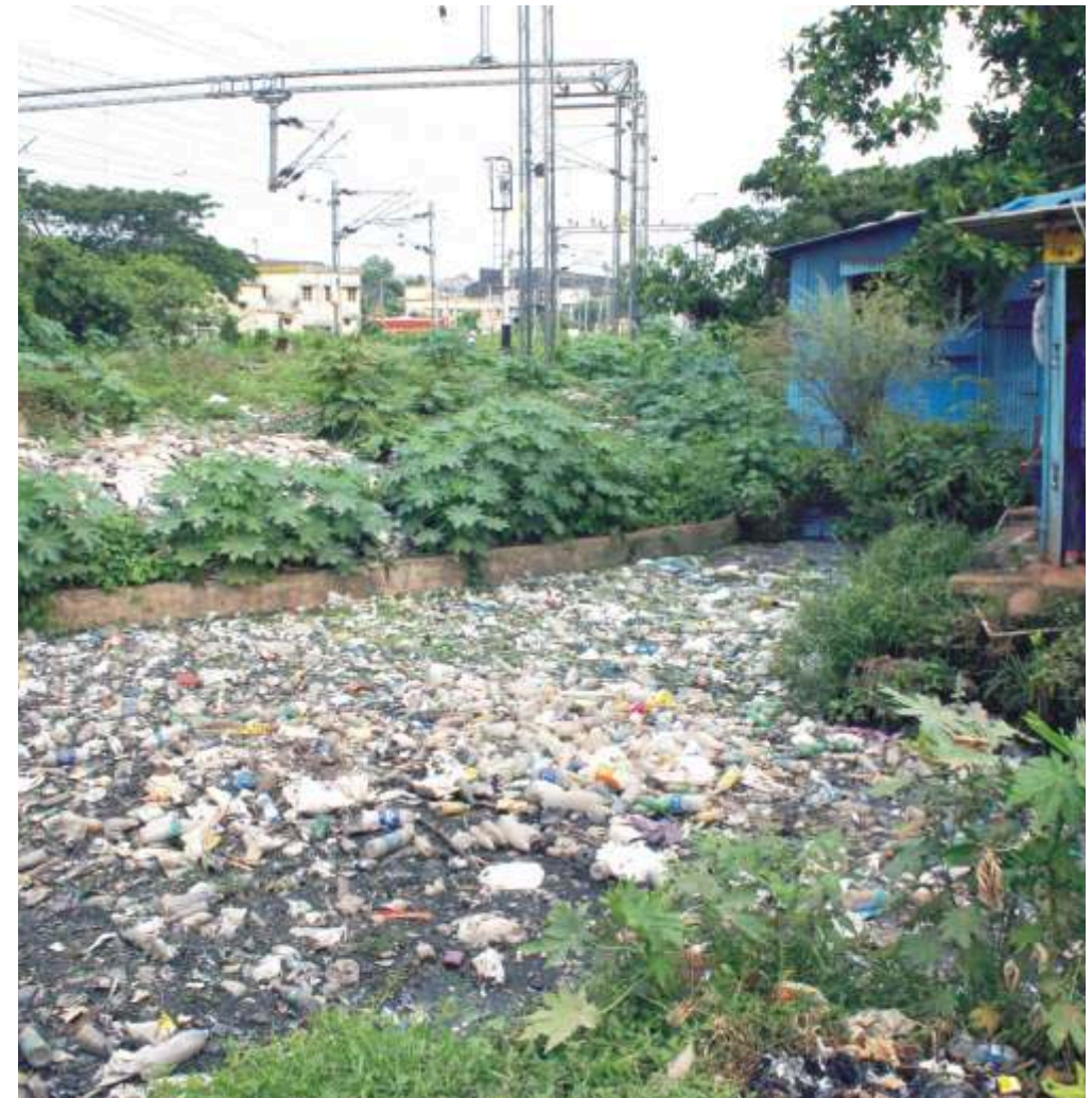
Figure 21: Garbage in open Drain
