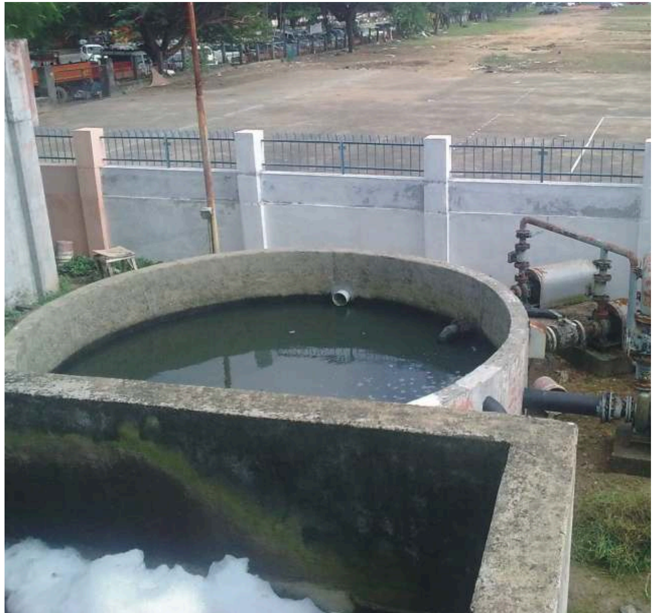
Figure 33: GCDA Sewage Treatment Plant at Marine Drive
