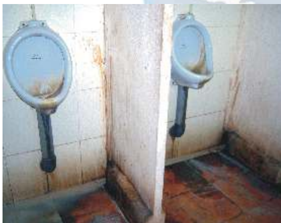
Figure 11(a): Poor condition of CTC
