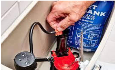
Figure 15.4: Tank bank to save on Toilet flushing
