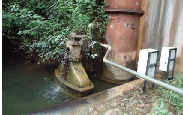
Figure 2: Leaking valve identified as a very high risk during WSP preparation
