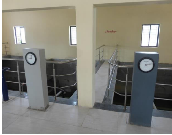
Figure 8.65: Rate of flow and head-loss indicator (Mechanical)
