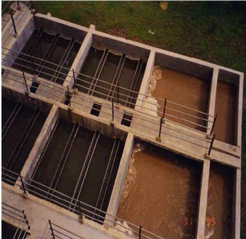
Figure 8.31: Performance photo at high turbidity (Tulsi, Mumbai, MCGM, Maharashtra)
