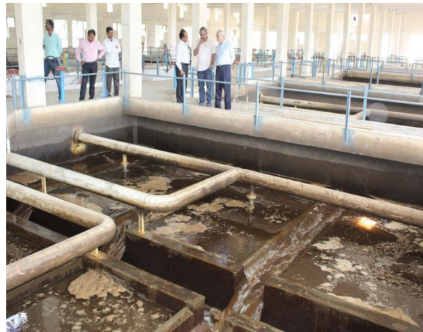
Figure 8.62: Filter bed during water (hard) wash operation
