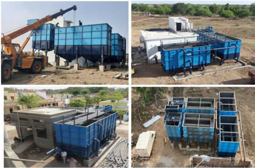
Pre-Fab Packaged Water Treatment Plants in Maharashtra ( Cap 0.50 to 3.0 mld)
