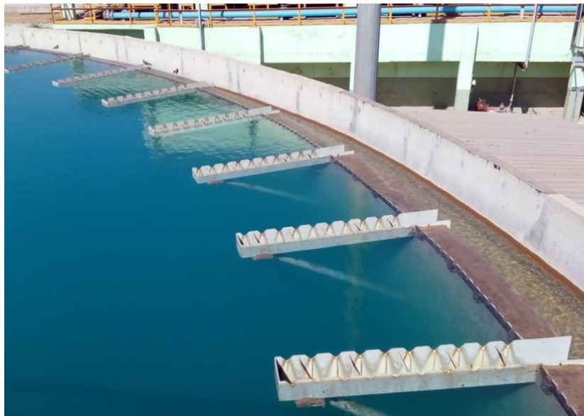
Figure 8.29: Finger weirs for Large Diameter Clarifiers/Clariflocculators in case they exceed weir loading
