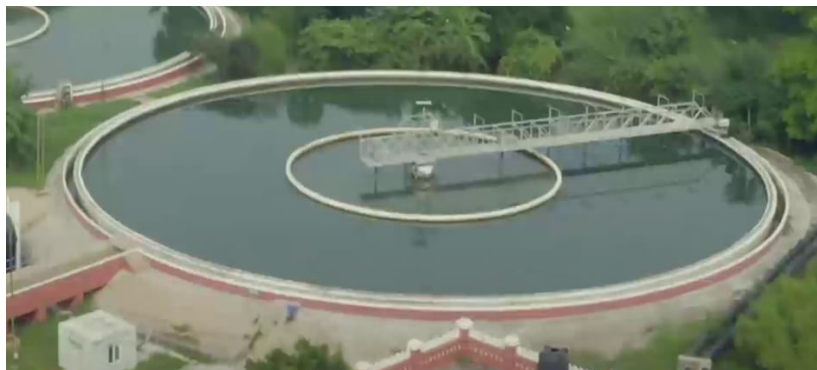
Figure 8.27: Flocculation zone with slow agitators & Clarification zone with scraper rotating bridge
