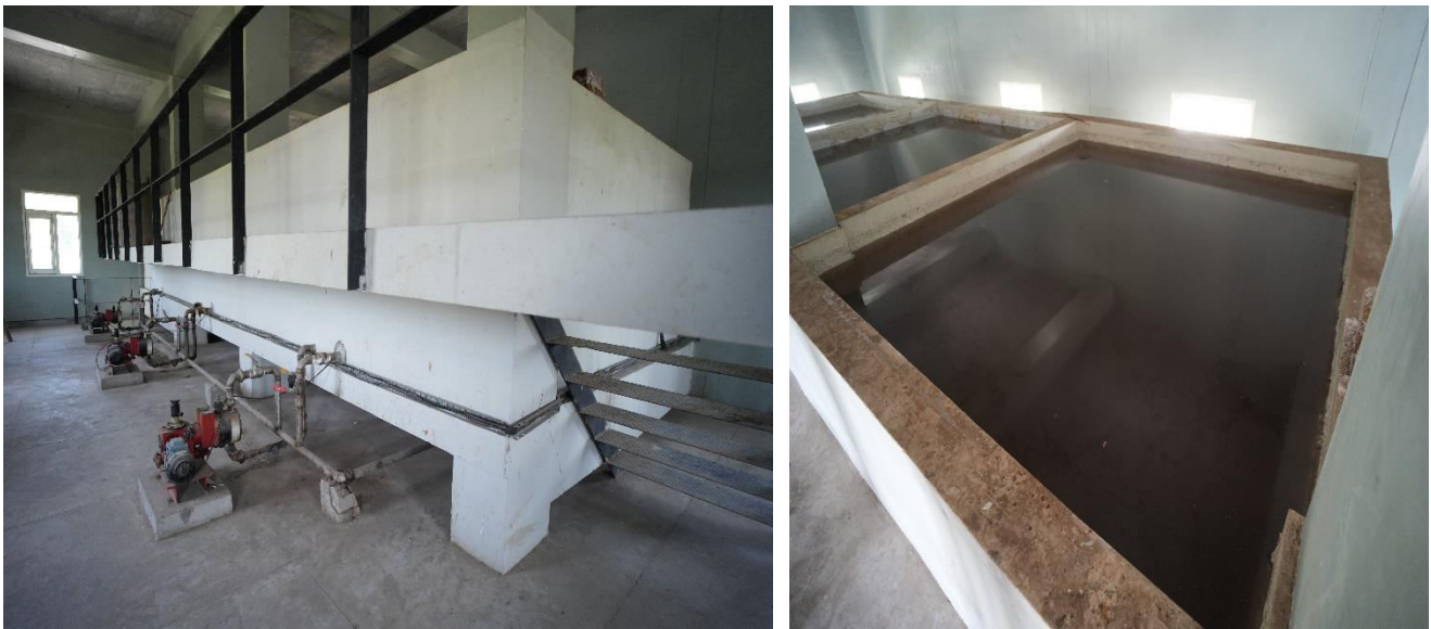
Figure 8.10: Solution Preparation tanks, Dissolving basket, and Agitator drive
