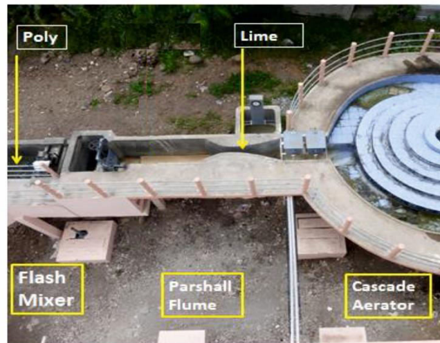
Figure 8.8: Dosing point locations in the WTP with Flash Mixer
