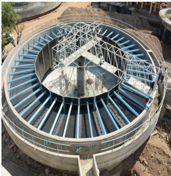
Figure 8.33: Clarisettler with rotating bridge scraper, WTP, Sangli, Maharashtra, Cap 80 mld
