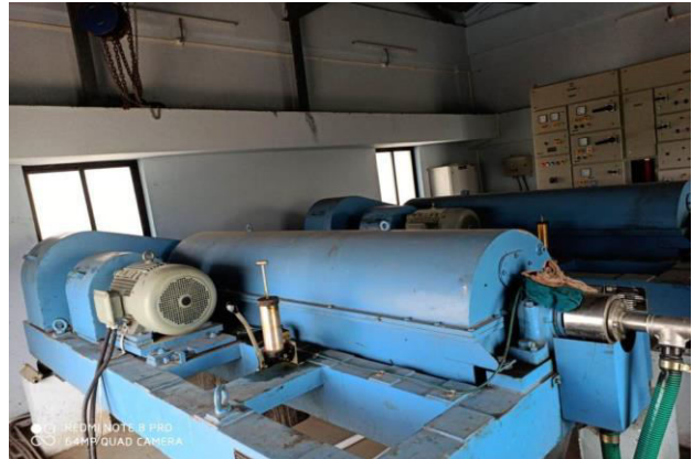
Figure 8.86: Centrifuges located on the first floor (source- Sangli, Maharashtra)
