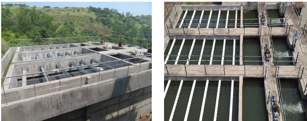
Figure 8.30: Tube Settling and flocculation under operation Modules & Troughs Capacity Plants, WTP at Pandharpur, Maharashtra
