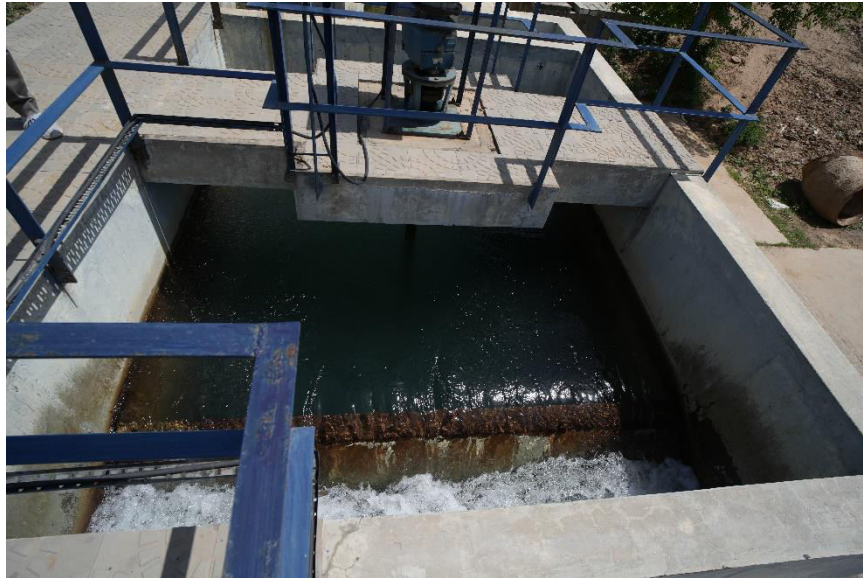
Figure 8.5: Rapid Mix Weir - Small Plant
