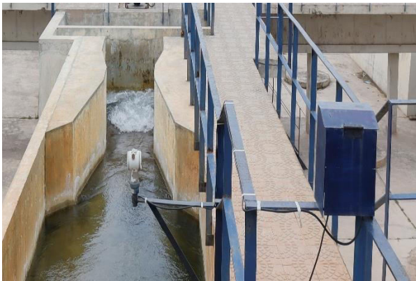
Figure 8.3: Ultrasonic Flow Indicator over Parshall Flume
