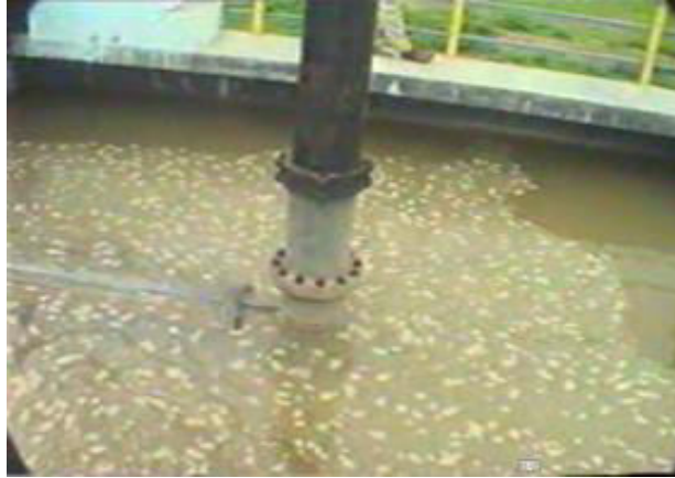
Figure 8.15: Floc formation at the top of the tank
