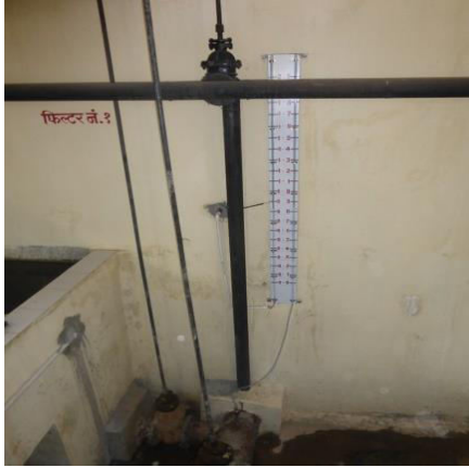
Figure 8.64: Headloss Indicator (Manometer)
