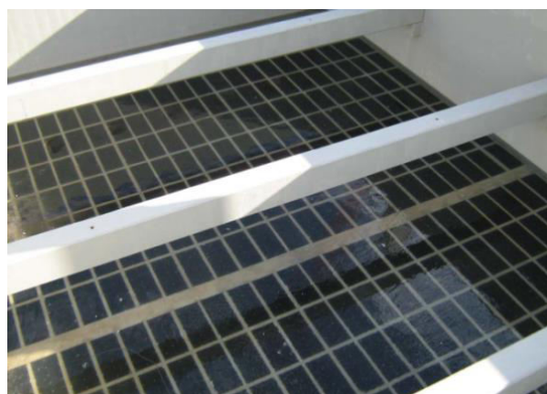
Figure 8.60: Filter floor with under-drain
