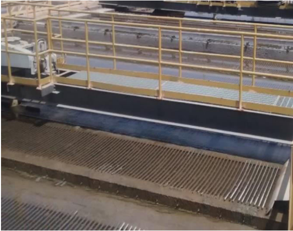
Figure 8.38: Plate Settlers at an Industrial plant (at Jamnagar in India)
