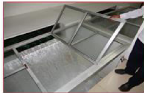
Filter Outlet Chamber with weir, Weir crest located above top of the media
