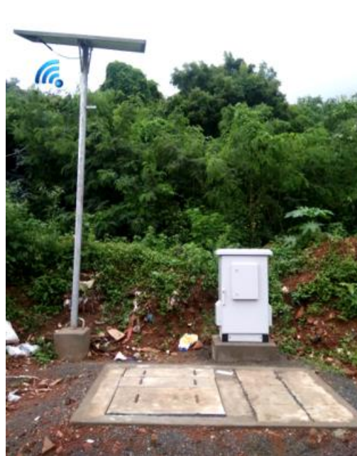
Figure 5: RTU at entry point of each DMA
