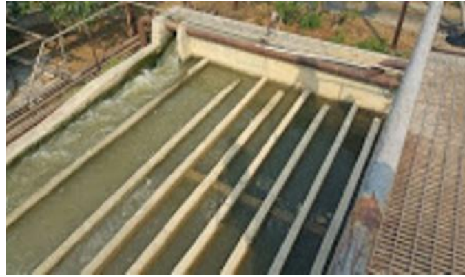
Figure 8.9: Horizontal Flow Baffled Flocculator
