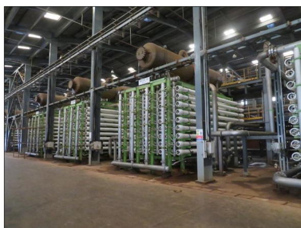
Figure 10.22: RO Membranes Skids
