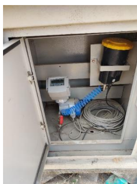
Figure 4: Bulk Flow Meter and pressure gauge at entry of DMA of Triveni OZ
