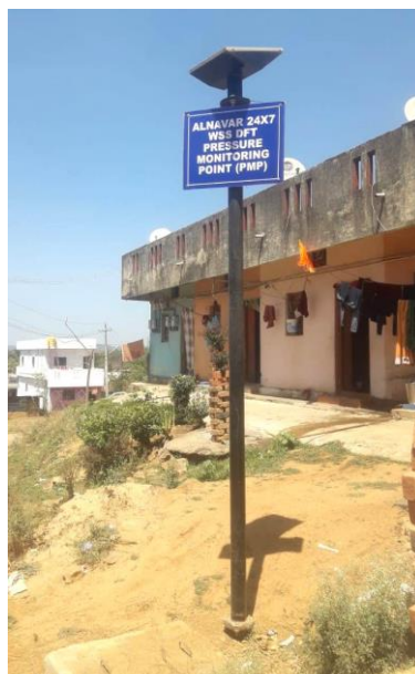
Figure 5: Online Critical Pressure Monitoring Point
