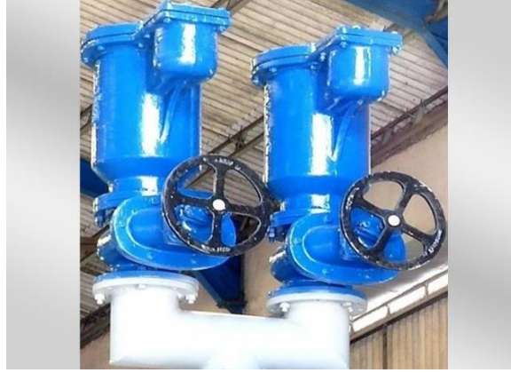
Figure 11.80: Double Chamber Kinetic Air Valve (Onsite)
