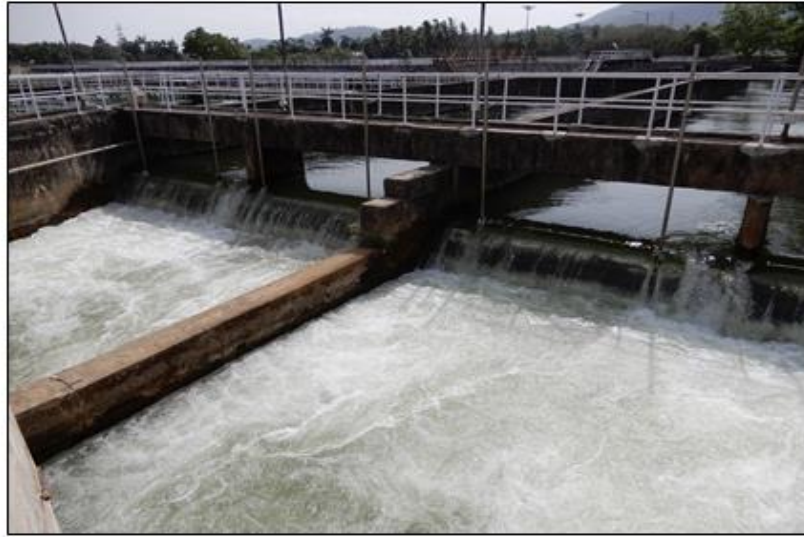
Figure 8.2: Weir Mixer (Rapid Mix Unit)
