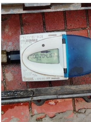
Figure 1: AMR meter at Ganesh Nagar
