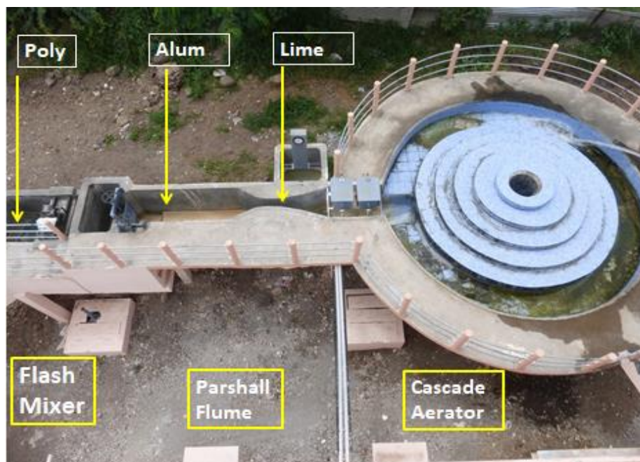
Figure 8.4: Dosing point locations in the WTP with Flash Mixer
