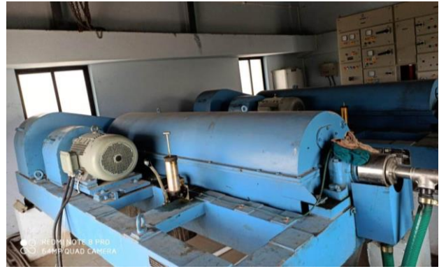
Figure 8.51: Centrifuges located on the First Floor
