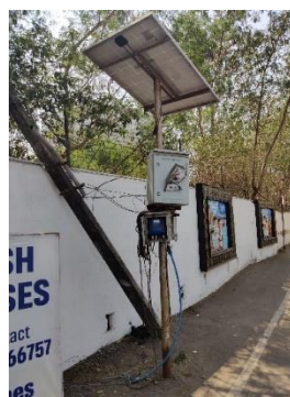
Figure 1: Bulk meters reader and transmitter
