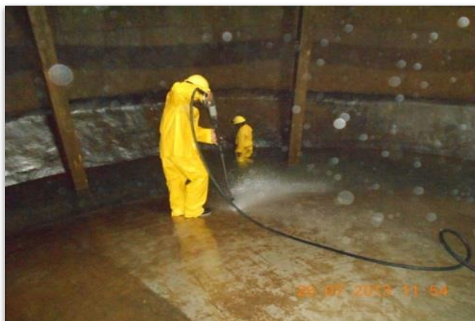
Figure 7: Tank Cleaning System
