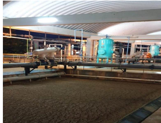
Figure 8.30: WTP at T K Halli, Bengaluru
