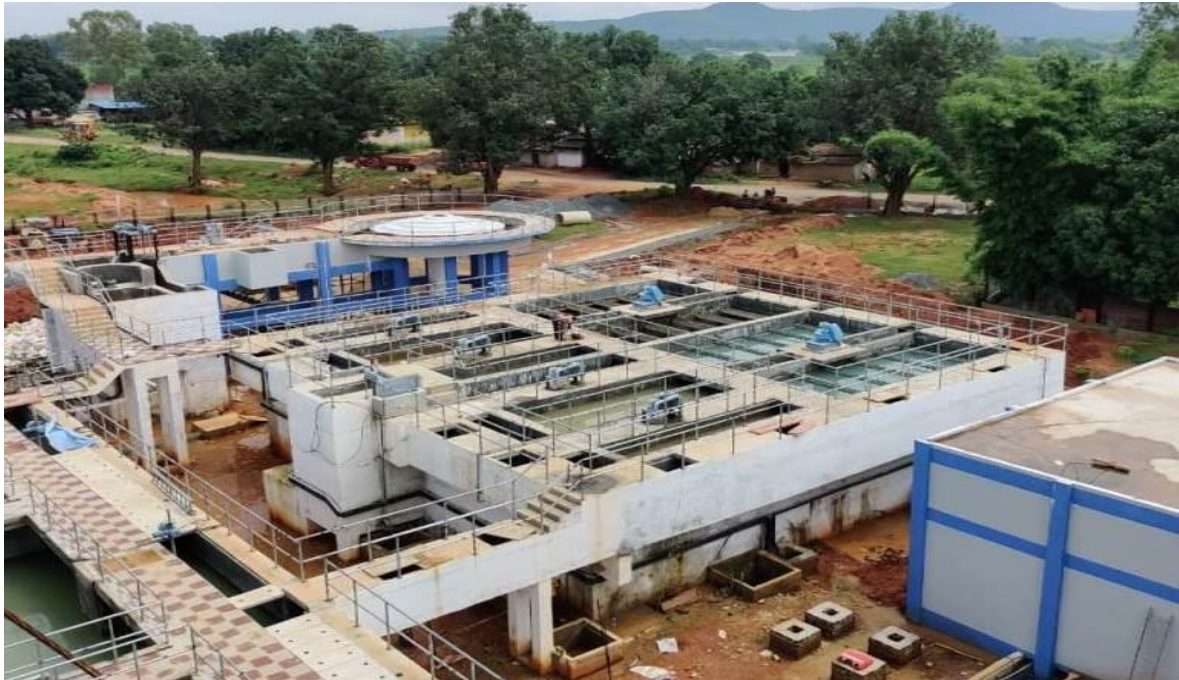
Figure 8.26: External Flocculators and Tube Settling Tank with Central Rake
