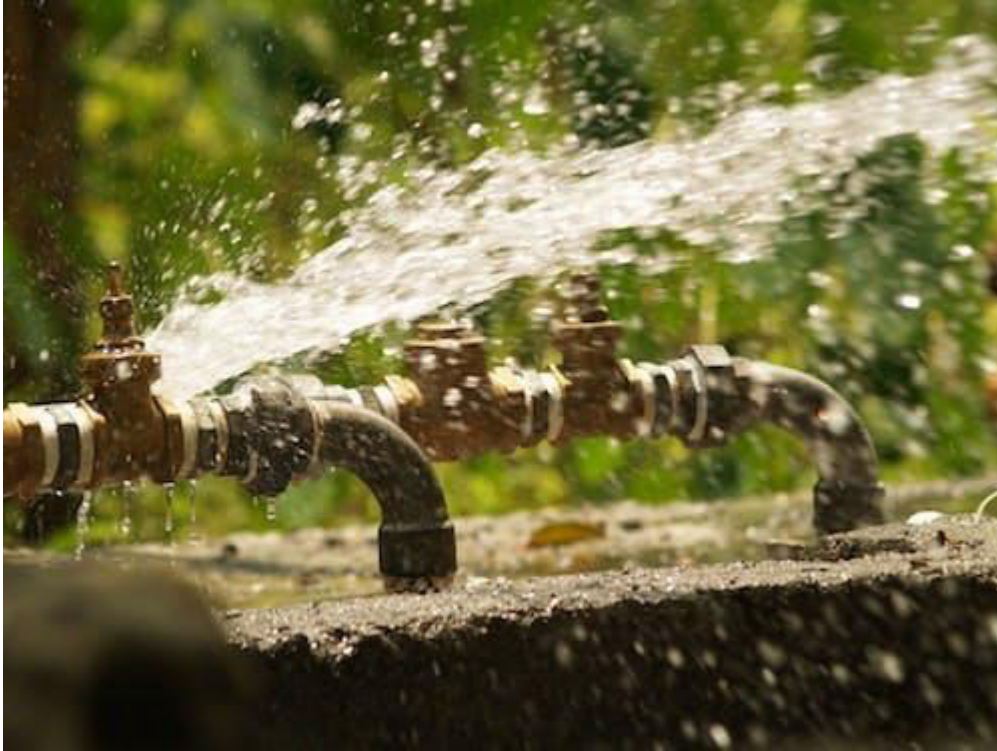
Figure: Typical leaks at a joint
