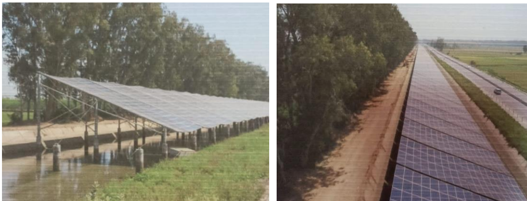
Solar Panels Installed on the Canals
