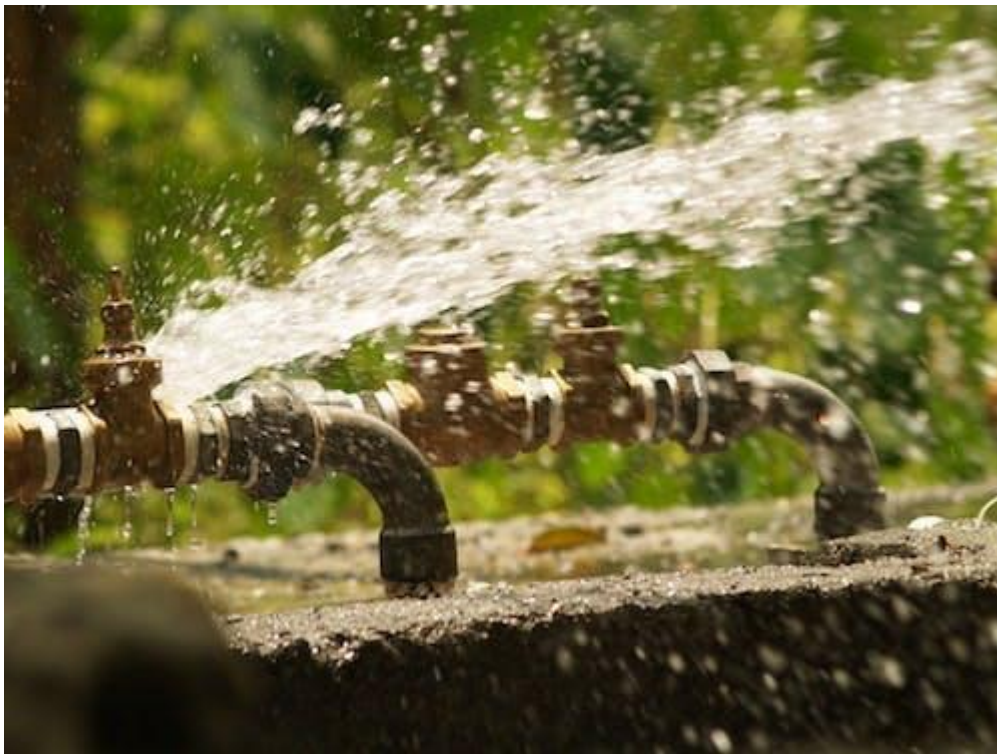
Figure11.2: Typical leaks at a joint
