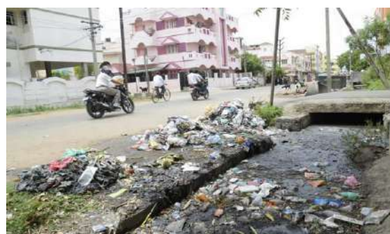
Figure 1.2: Dumping of Solid Waste in Storm Water Drains
