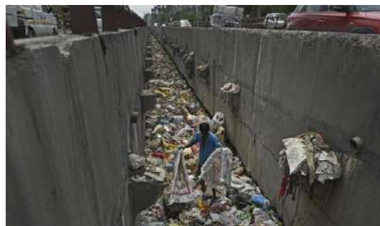
Figure 1.5: Plastic in Storm Water Drain
