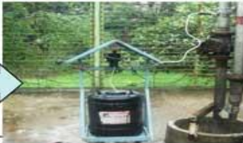
Chlorination arrangement - Dosing pump
