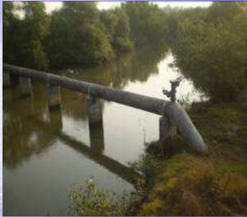
Clear water Transmission Line
