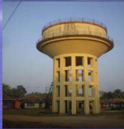
Zone I OHT of 5 Lacks Capacity
