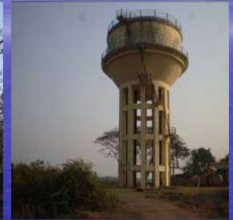
Zone III OHT of 5 Lakhs Capacity
