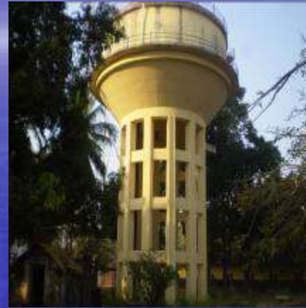
Zone II OHT of 5 Lacks Capacity
